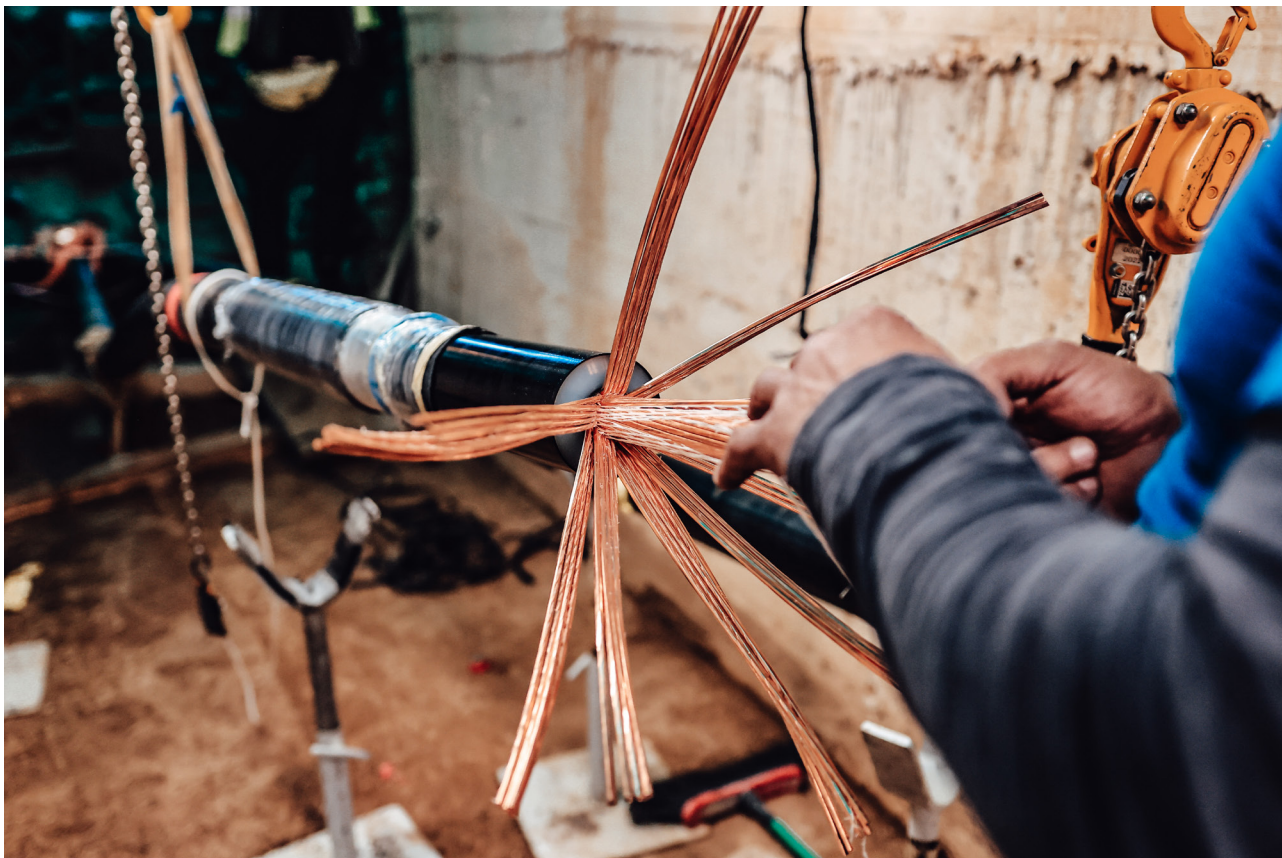
The second interconnector significantly strengthens security. With a nominal capacity of 225MW, development permits in Malta and Italy have been achieved, and construction is underway.
